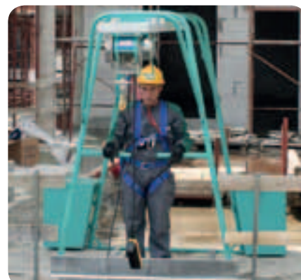
Gantry for stand hoists
