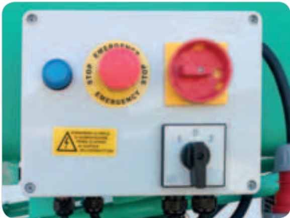
Tph Machine Control Panel
